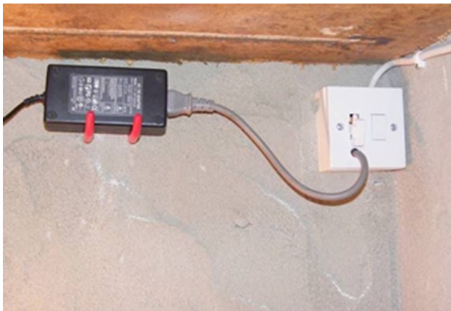
Figure 11-11. The 12V DC power supply
